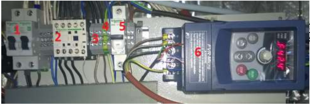
d Board. verter SIEMENS (0,37KW)
